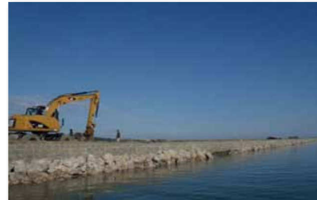
The same embankment after the reconstruction works provides for flood protection in the hinterland
