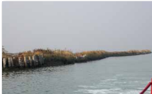
The embankment that has not been maintained for years cannot defy the increasingly higher tides
